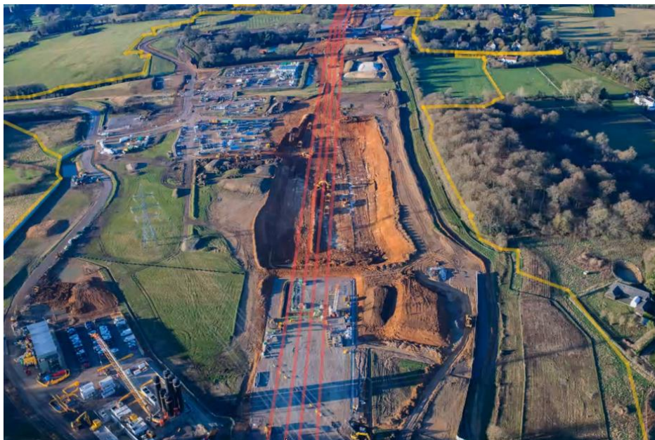
Excavation at South Heath, showing the area in the foreground in which 'barrettes' will be sunk and the start of the cuttings heading north
